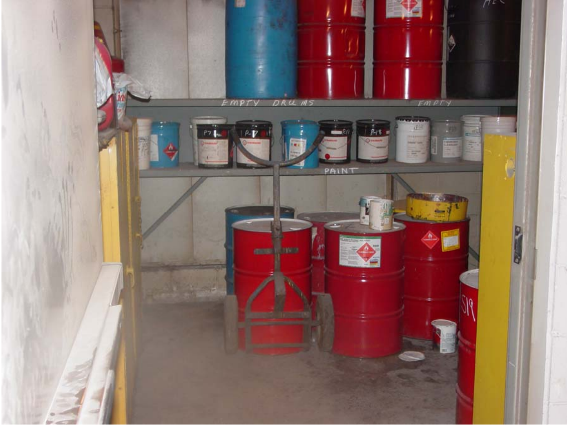
Explosion proof room and exterior wall with blow out panels.
