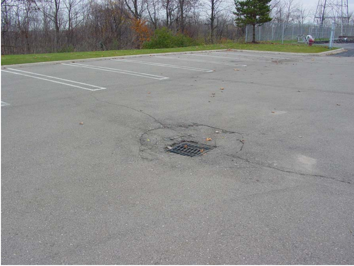
Catch basins need concrete collars and repairs.
