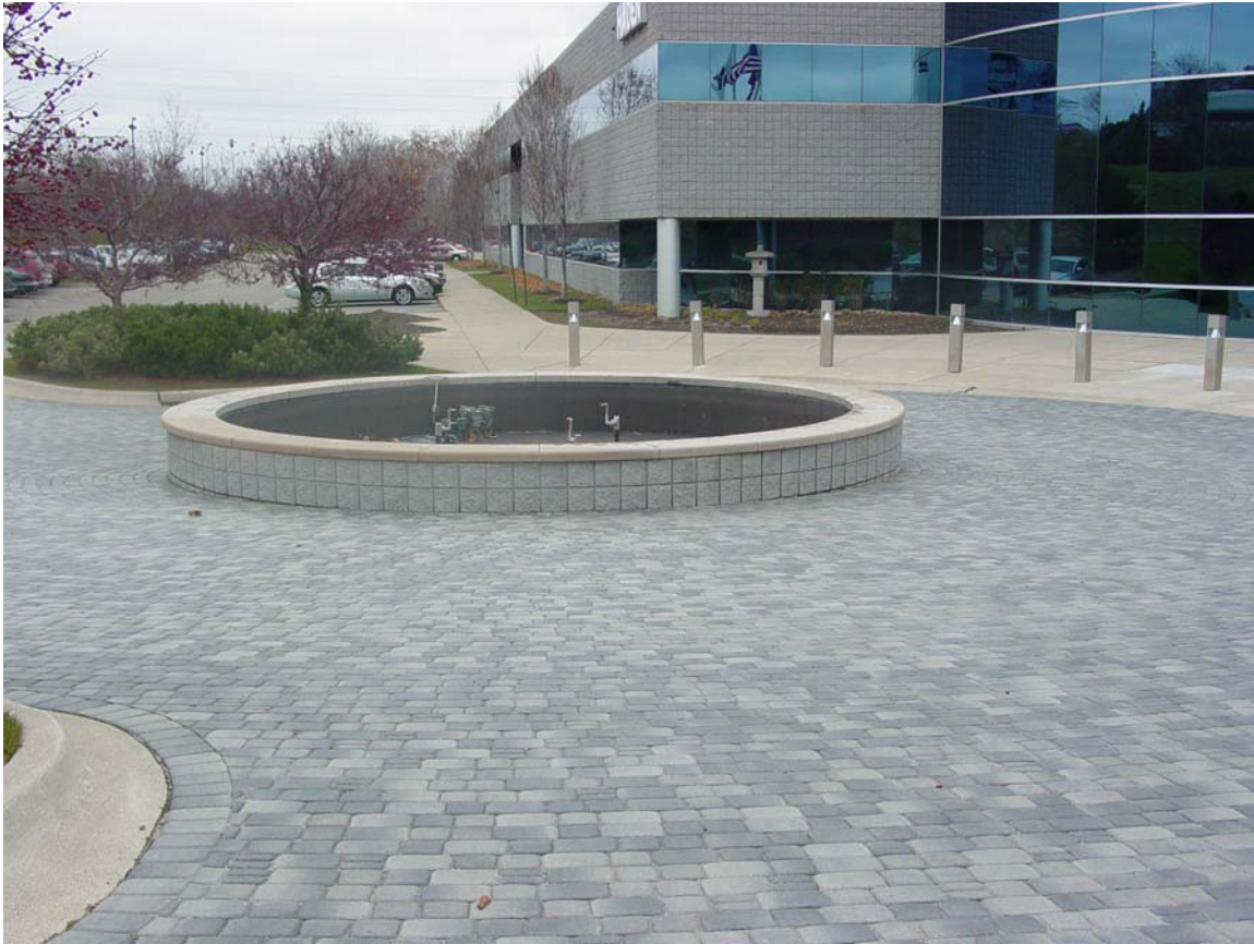
Fountain and brick paver drive. Fountain being worked on 2005 and pavers replaced in 2003/4 for deterioration from the bottom side.
