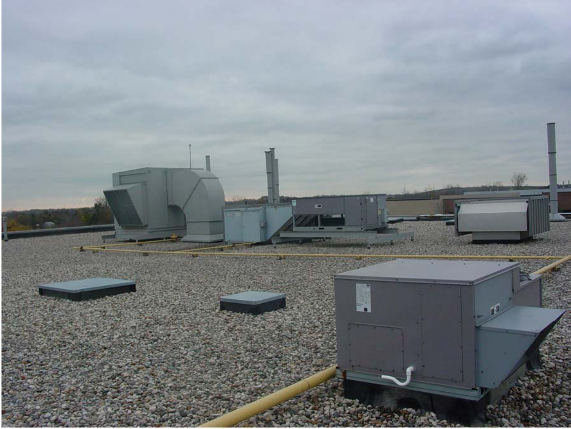
Roof top mechanical.
