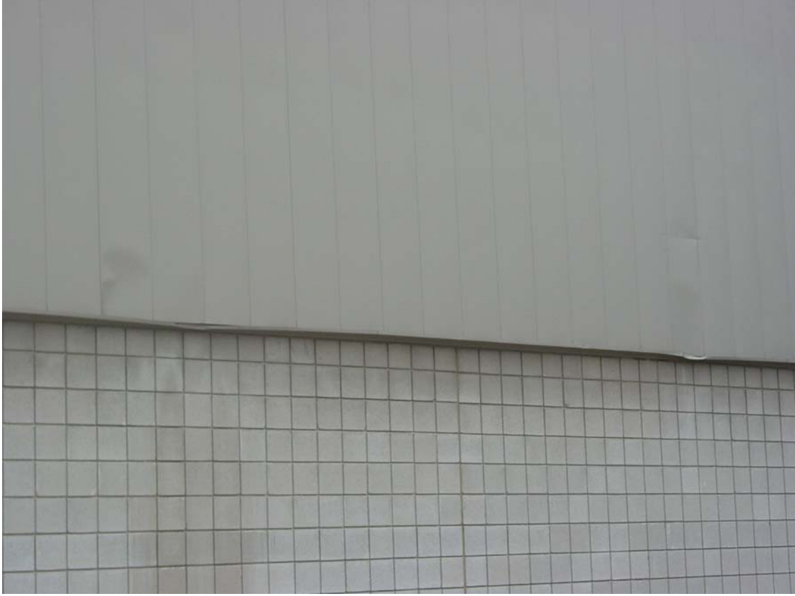
Minor damage to metal siding.
