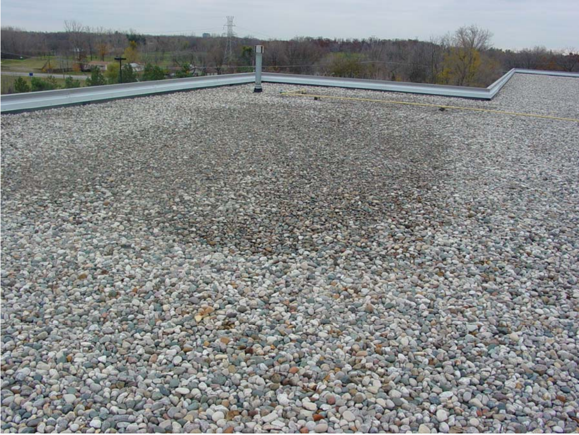
Roof - areas of water ponding.
