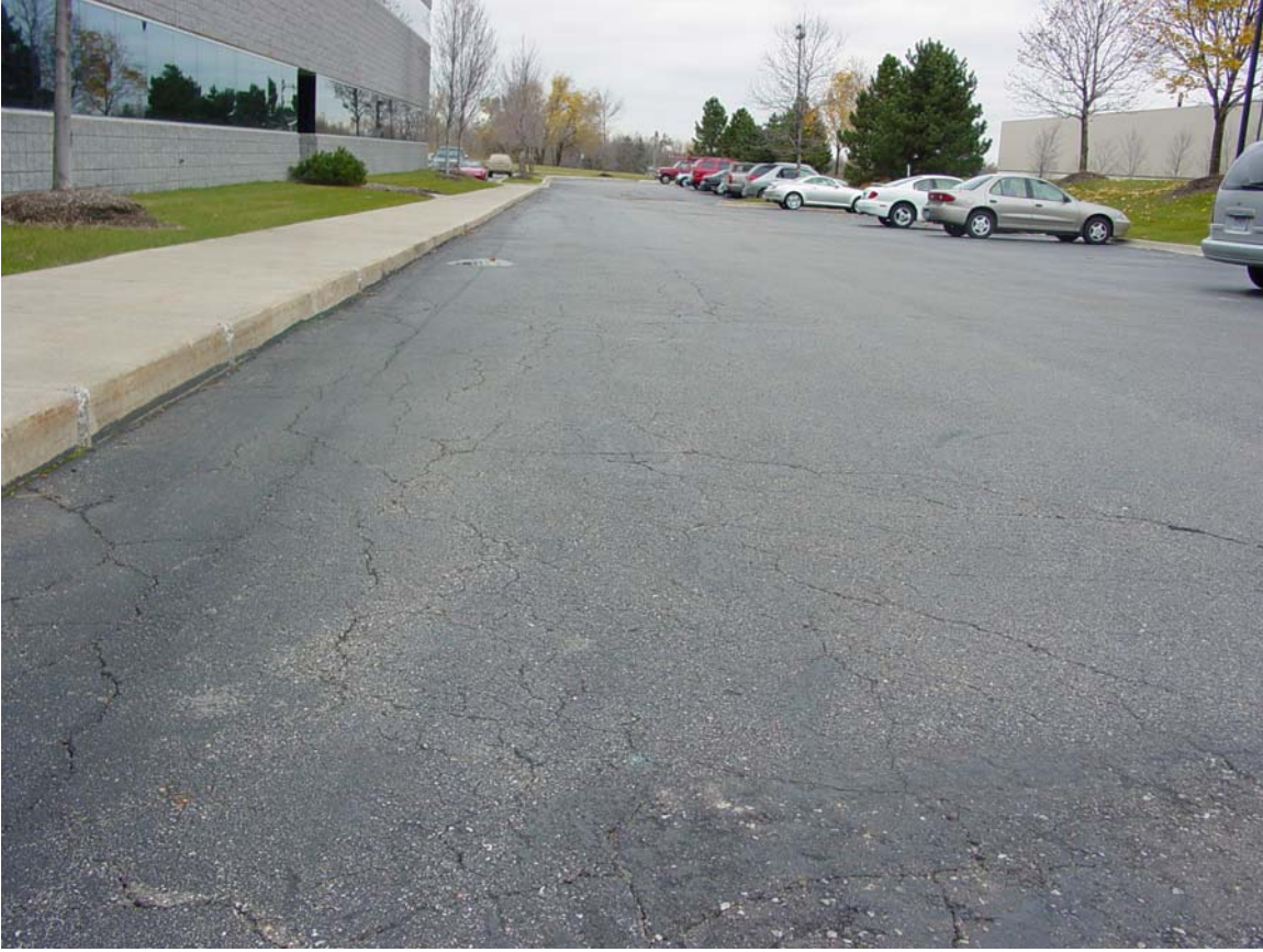
Condition of asphalt needs sealant and repairs. Cracking and tire groves.
