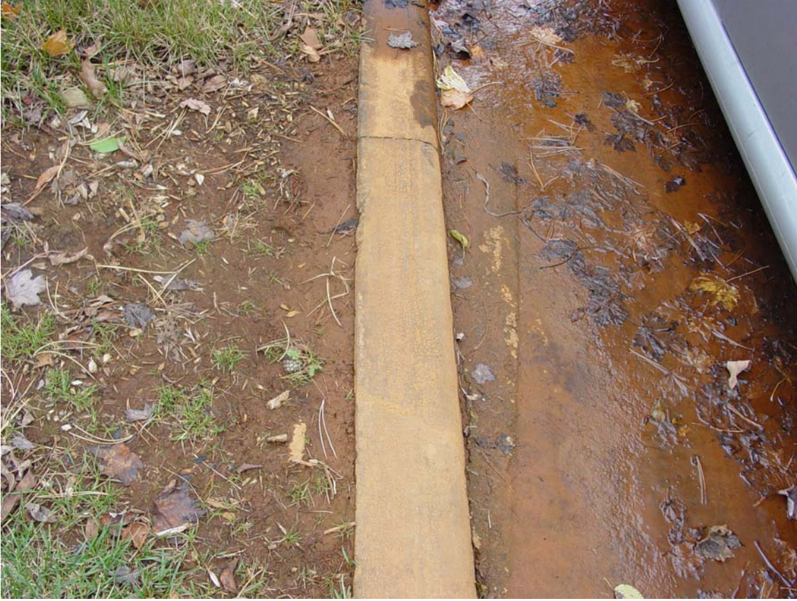
Iron deposits on concrete curb, asphalt, and ground.
