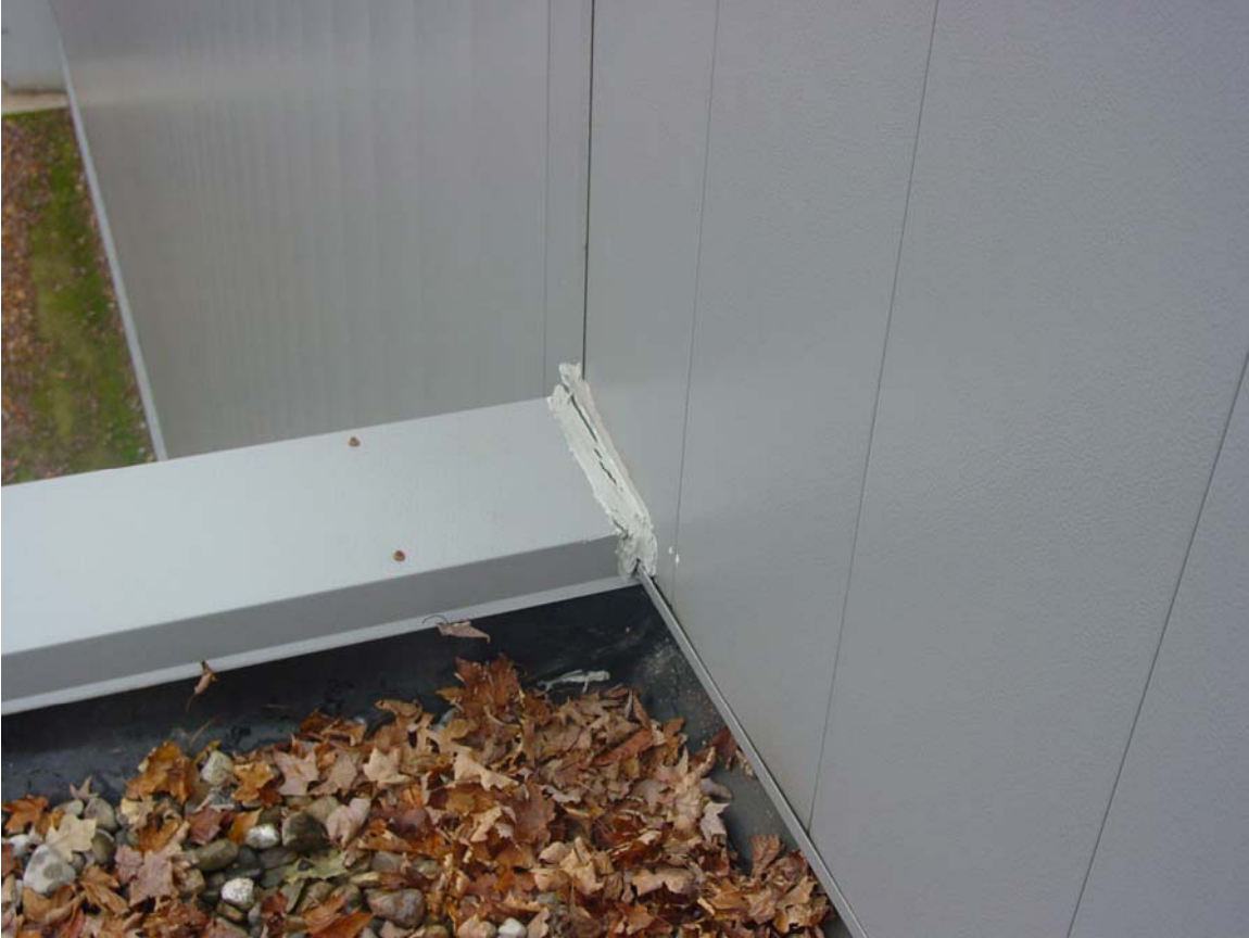
Roofing material showing signs of shrinkage.
